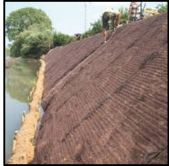
This is an example of erosion control, tarps are placed over a stream bank to help stop water erosion.
